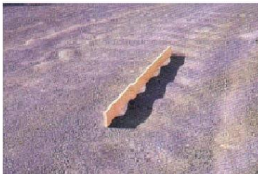
Gambar 2.8 Retak Keriting ( Corrugation )
