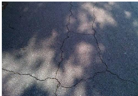
Gambar 2.2 Retak halus ( hair cracks )
