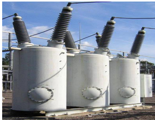
Gambar 2.4 Oil Circuit Breaker
