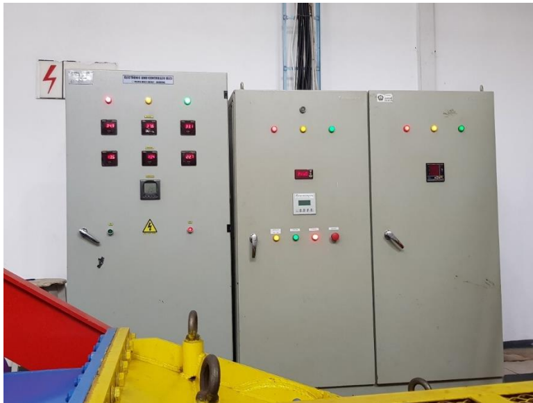
Panel Electronic Load Controller (ELC)
