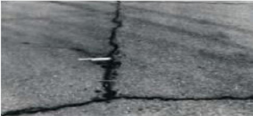
Gambar 2.19 Retak Sambung (Lane Joint Cracks)
