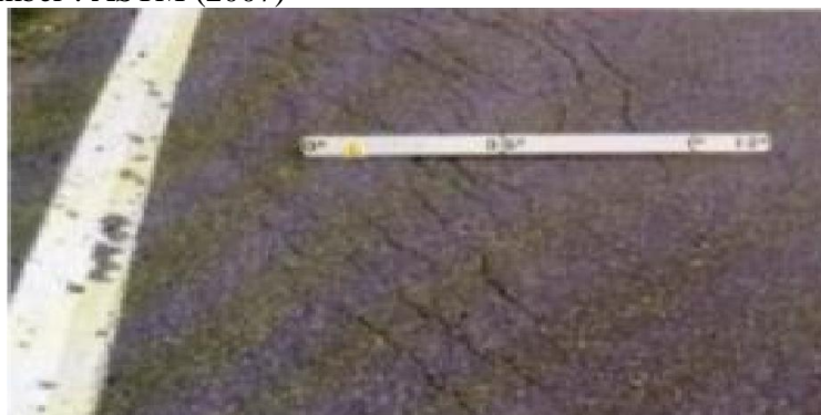
Gambar 2.37 Patah Slip (Slippage Cracking)
