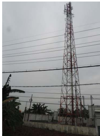
Gambar 4.2 Tower Greenfields PT Telkomsell
