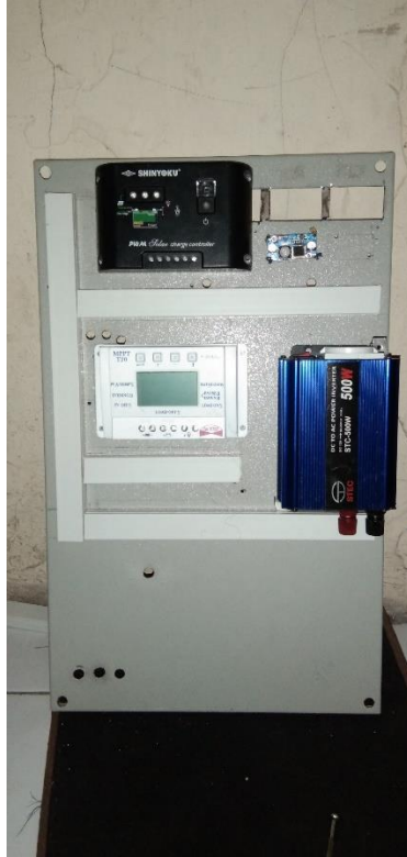
Foto control panel box
