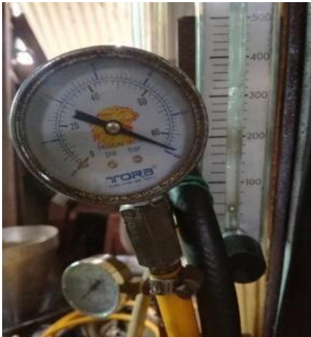
Pressure gauge dan Flowmeter
