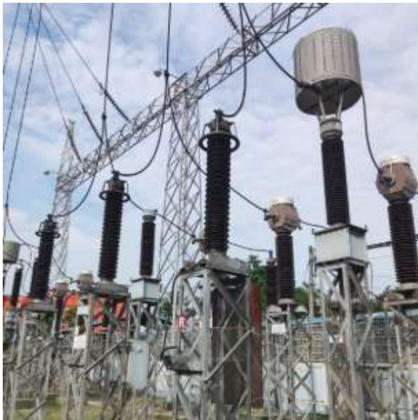
( Monitoring Lokasi Swict Yard )
