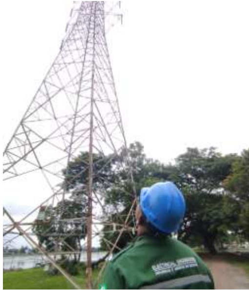
( Monitoring SUTT 150kV )
