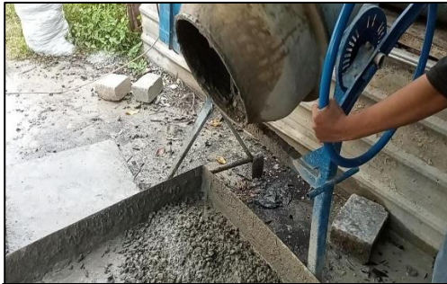
Concrete admixture shedding
