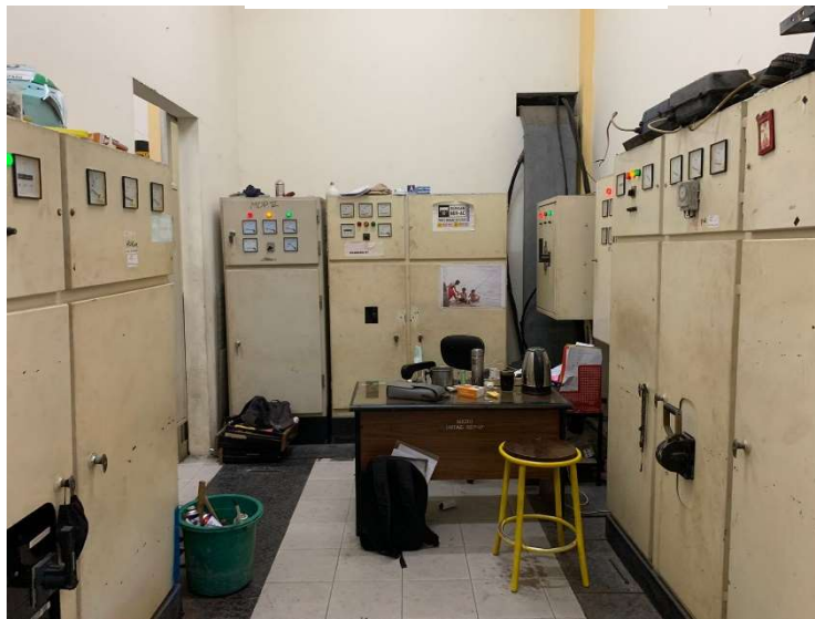
Gambar Ruang Genset
