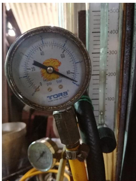
Pressure gauge dan Flowmeter
