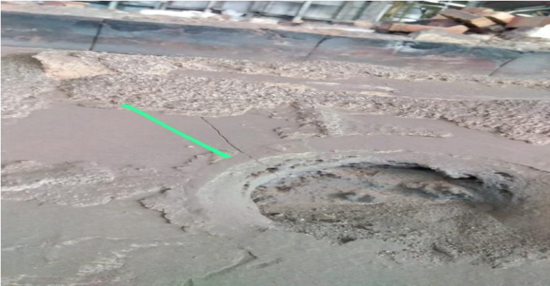
Lampiran 8. Gambar Cacat Crack
