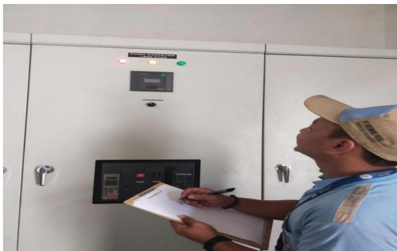
Gambar pengambilan Data di MDP ( Main Distribution Panel )
