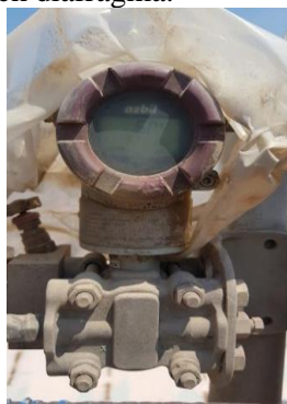
Gambar 6. Pressure Transmier 32-PT 801
