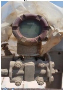
Gambar 6. Pressure Transmier 32-PT 801
