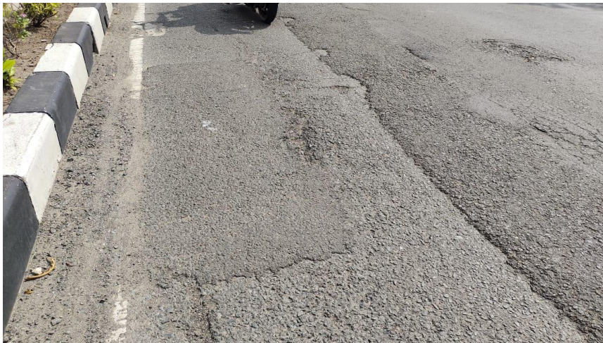
Figure A 6 Patching (Source : Reseacher Data, 2022)
