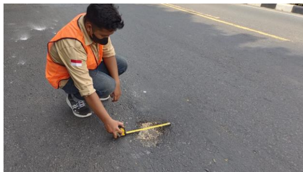
Figure A 11 Calculation Area of Damage (Source : Reseacher Data, 2022)
