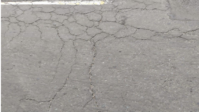
Figure A 1 Alligator Cracking (Source : Reseacher Data, 2022)
