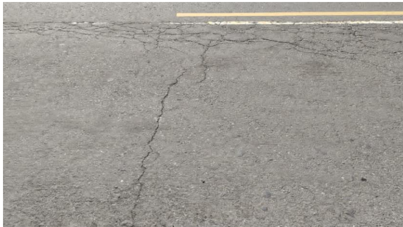
Figure A 2 Transversal Cracking (Source : Reseacher Data, 2022)
