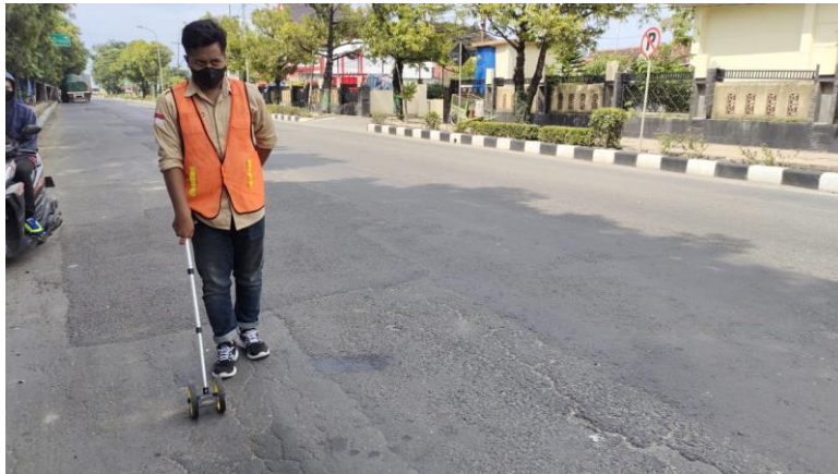
Figure A 9 Measurement of Road Damage Length (Source : Reseacher Data, 2022)
