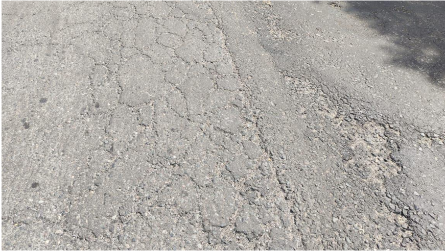
Figure A 7 Random Cracking (Source : Reseacher Data, 2022)
