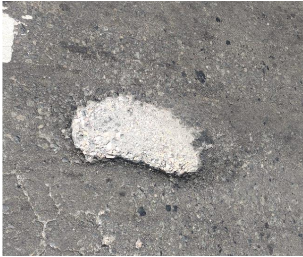
Figure A 3 Potholes (Source : Reseacher Data, 2022)
