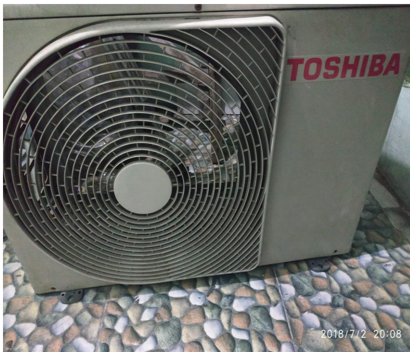
Gambar 3.4 : Mesin Pendingin Air Cooler 1PK
