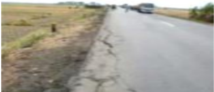
Gambar 2.5 :Retak Pinggir (Edge Cracking)
