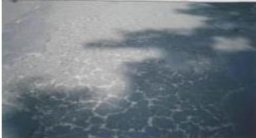
Gambar 2.13 : Pelepasan Butir (Weathering/Raveling) Sumber: Bina Marga NO.03/MN/B/1983
