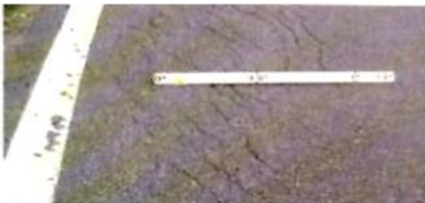
Gambar 2.4: Retak Selip (Slippage Cracking)
